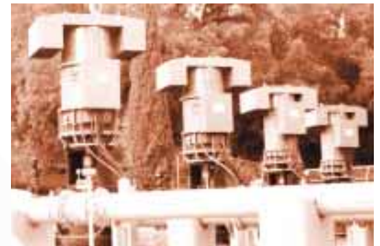
Medium voltage water pumps
