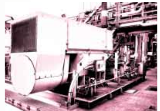
Water injection pump on board an FPSO
