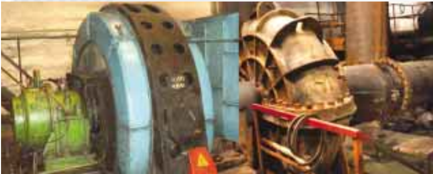
Synchronous motor driving an iron ore pump
